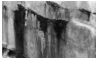
Figure 9 – Evident corrosion of the metal rod in the reinforced concrete
